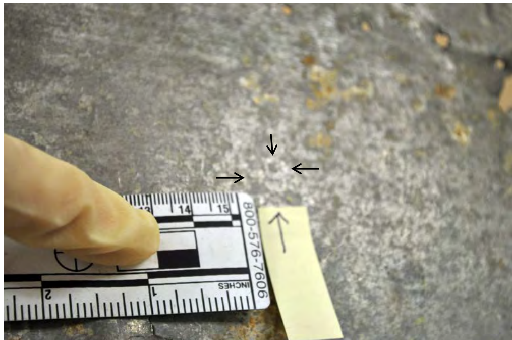
Figure 9: An apparent "-9" near the Sta. 307 feature, arrows.
